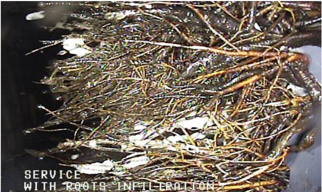
Figure 2. Photo of the interior of sanitary line displaying service line connection with roots and infiltration.
