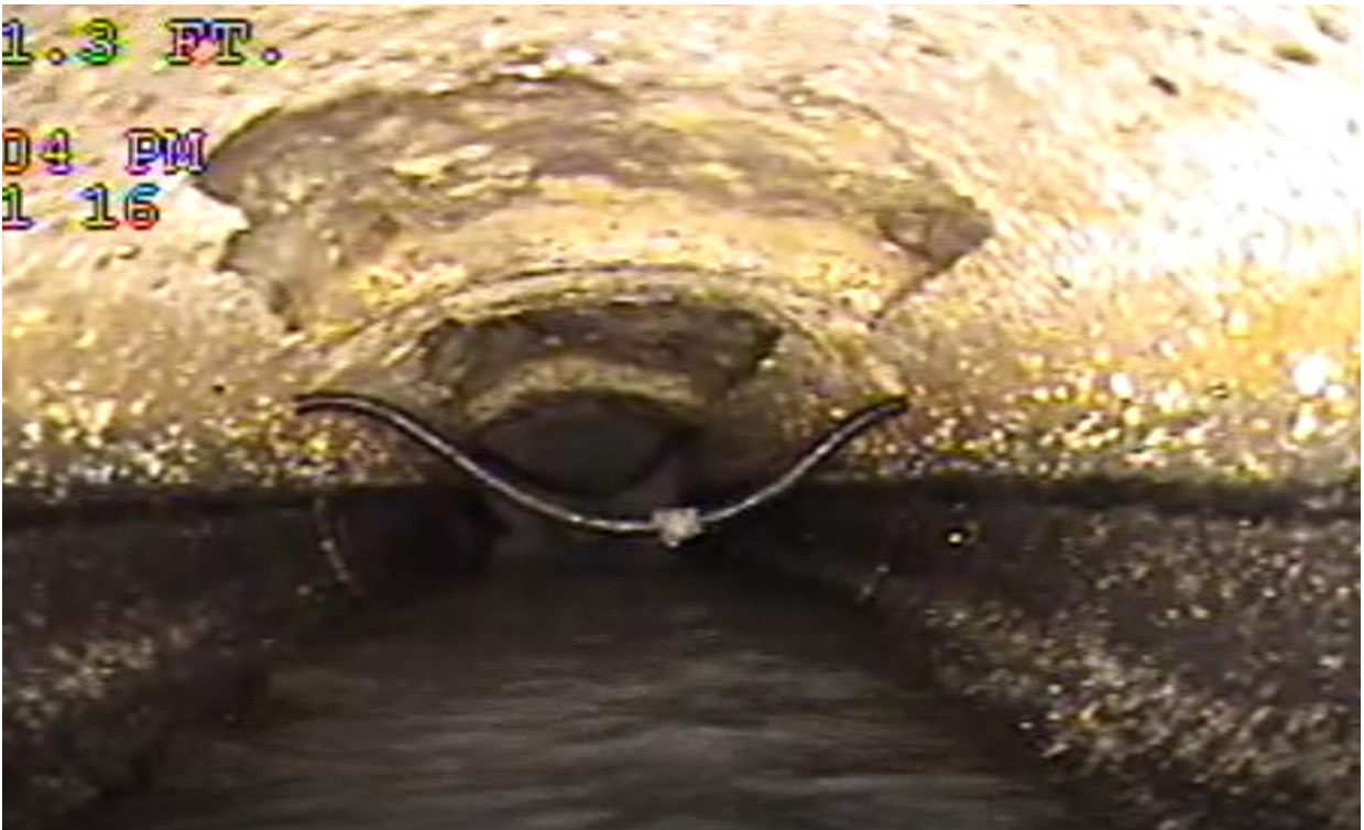
Figure 3. Photo of the interior of sanitary sewer pipe showing degradation down the line and gasket failure.
