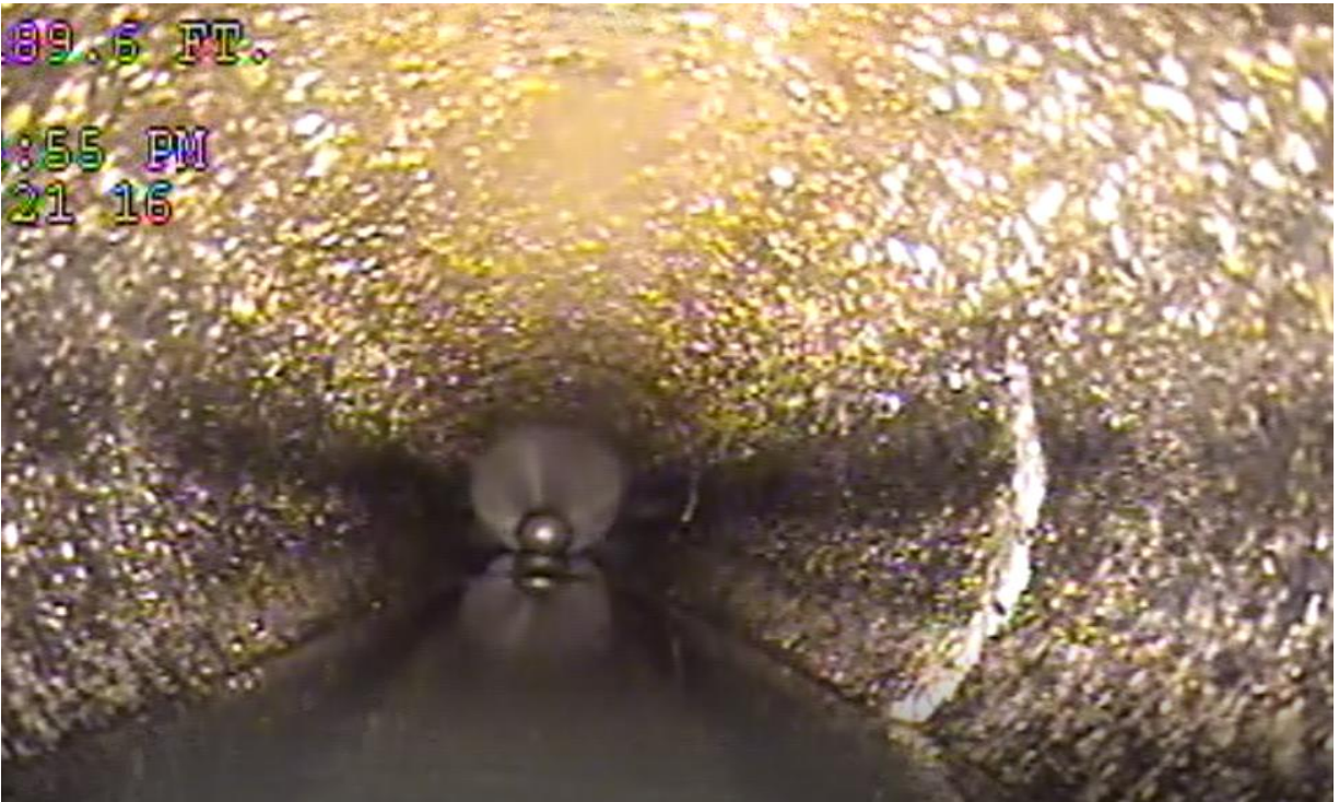
Figure 1. Photo of the interior of sanitary line displaying exposed aggregate.
